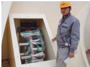
Mr T. S. Kim opens a hatch showing Roxtec installations for secure cable routing onboard LNGC Carriers.
