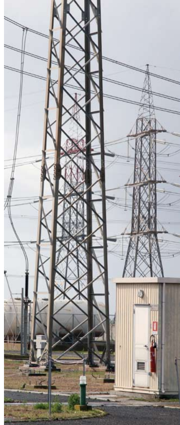
Roxtec seals the cables that enter the control boxes at the substation.
