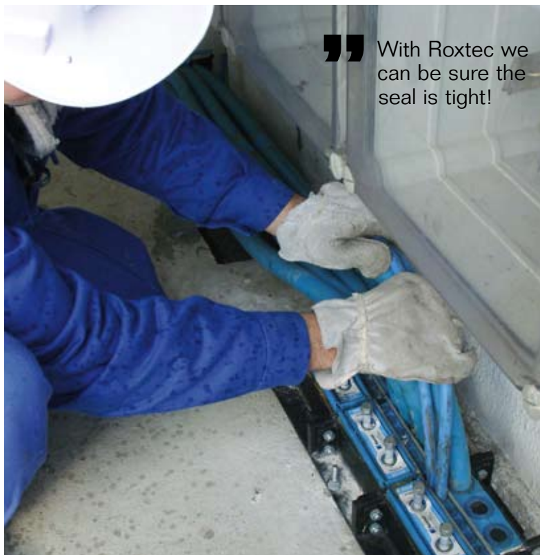
Roxtec seals cables in a manhole outside of the control room. Spare capacity has been added with extra seals for future cables.
