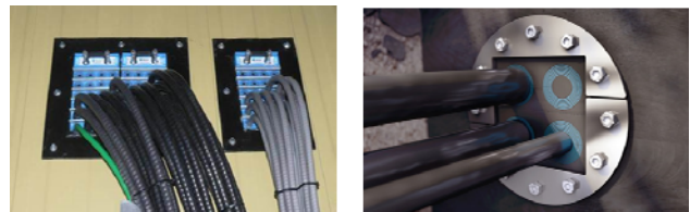
Fig. 9 Shows use of multi cable transit devices to provide vaportight barriers where cables or pipe enter buildings
