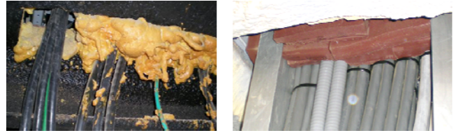
Fig. 7 Example of cable entries which have been compromised
