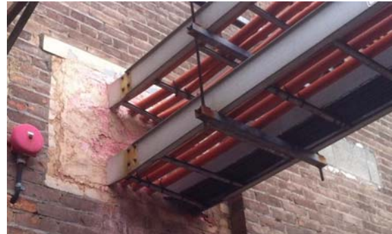
Fig. 8 Example of the use of compound as a vaportight barrier to seal the opening of cable entry.
