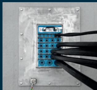
MV and LV power cables
