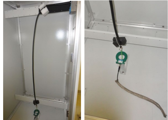
Fig. 8. Views of the coaxial cable inside the cabinet; pieces of foam are used to separate the cable from metallic parts; the Pearson current sensor is placed near the base of the cabinet; the braided shield for the current sensor cable is bonded to the cabinet at the point it enters, from below.
