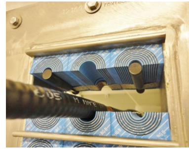
Fig. 7. Sealing and bonding modules of the Roxtec BG™ cable transit used in Case 3; the outer conductor of the coaxial cable makes contact with the frame by means of a meshed arrangement of large and short braids.
