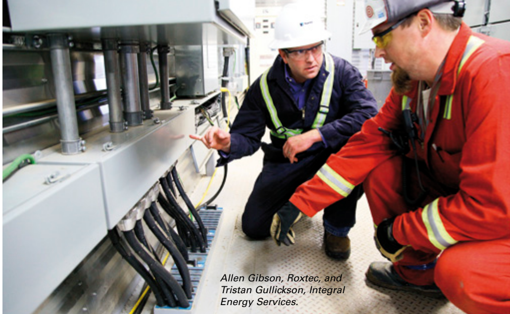
Roxtec seals in the floor of the control center.
