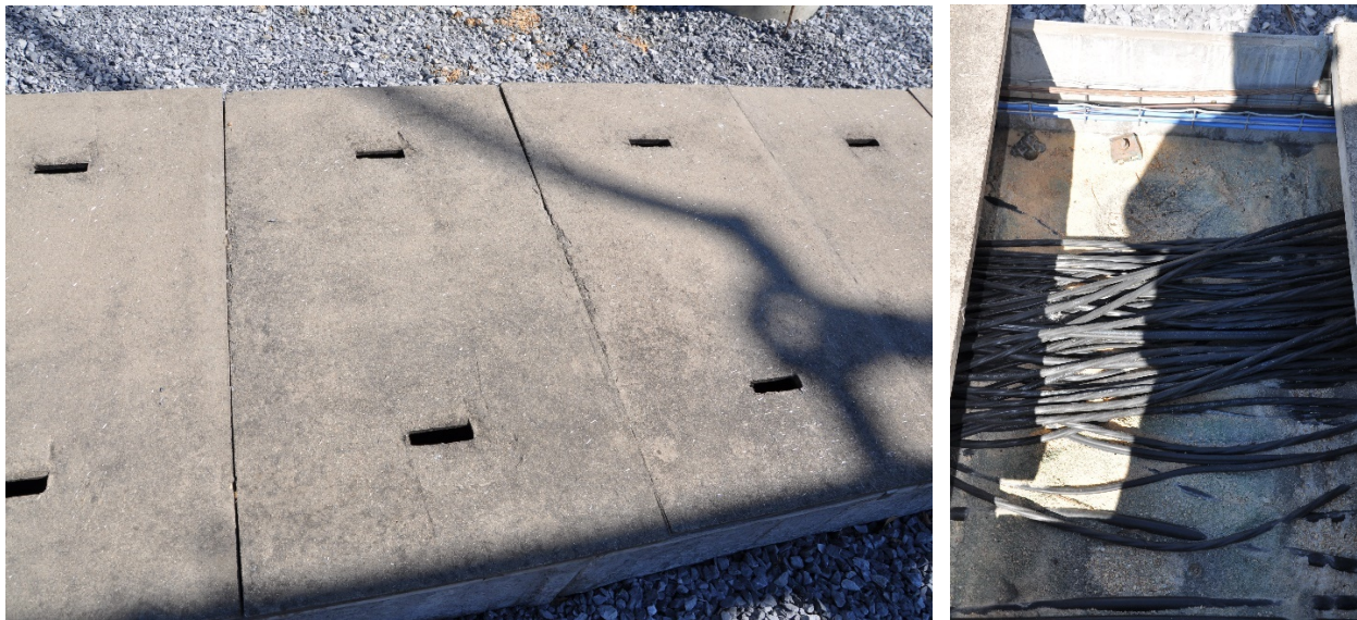
Figure 5-6 Example of a cable trough located within a substation
