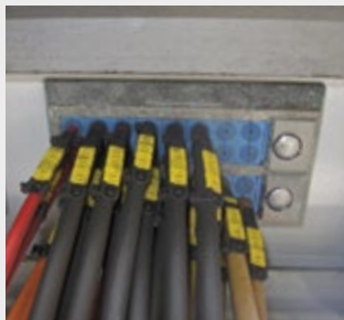
Field-based junction boxes
