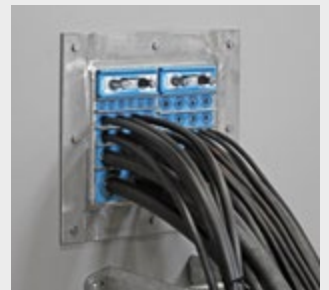
Motor control centers
