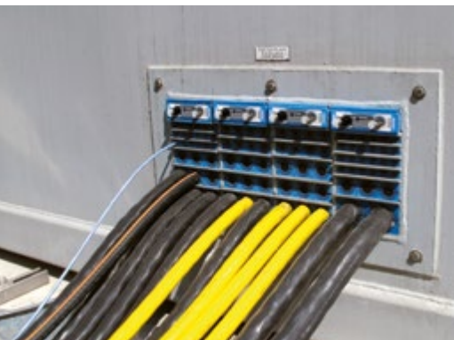
Bolted Roxtec SF frame
