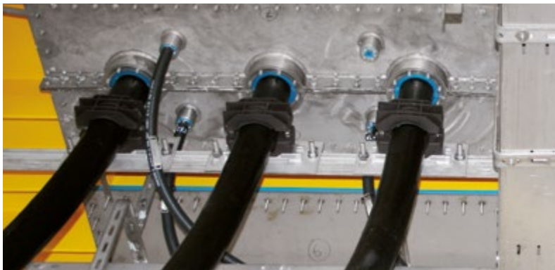
Openable steel plates with cable seals for transformers
